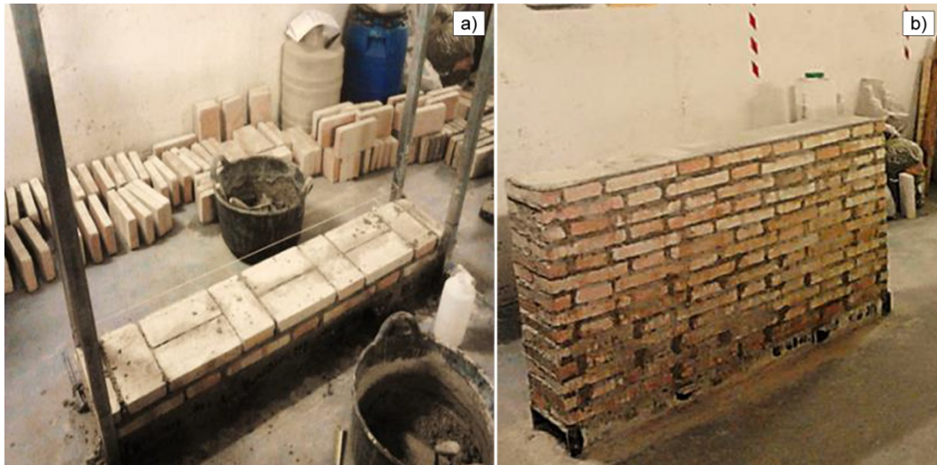
Figure 10 - Historical-like wall built at UPC: construction stage (a) and the wall at the end of the construction (b).
