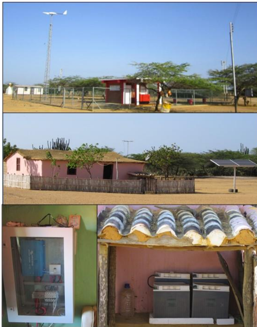
Figure 3. Microgrid (top), individual system (center) and inverter/battery (bottom) in Jacuque, Venezuela
