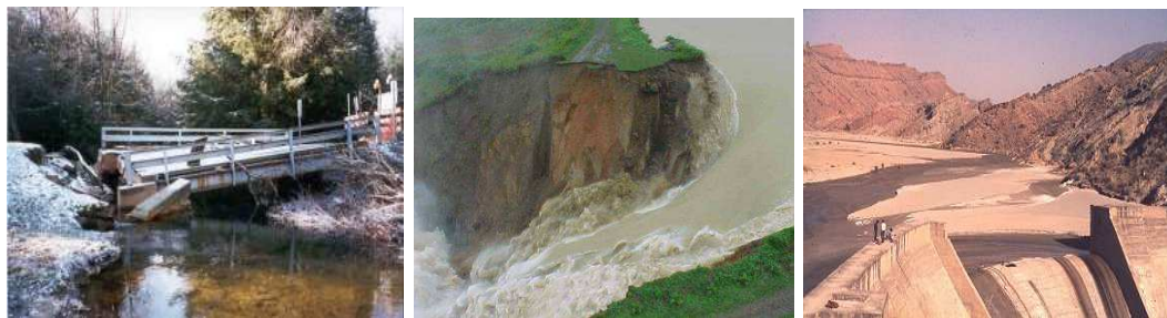
Figure 2. 1. Sediment transport effects: a) Infrastructure damage; b) Bank erosion and c) Dam silting up (after Haynes, 2011).
