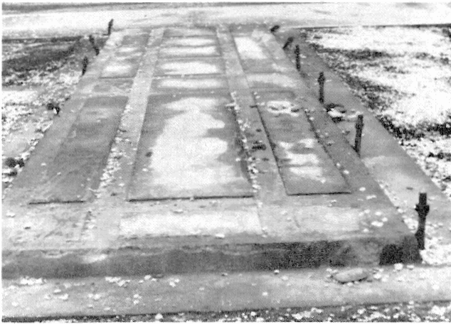
Figure 2. A Properly Grouted Platform which Later was Removed from its Concrete Pad. Note that 100% Contact had been Obtained by the Grout on All Longitudinal and Transverse Supporting Beams.
