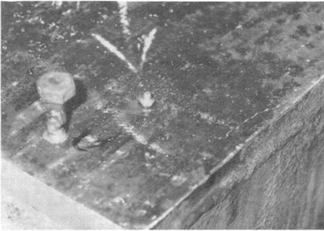
Figure 12. A Close-up View of One Injection Site. Injection Sites were Installed at Each Corner of the Gear Box Support Shown in Figure 7.
