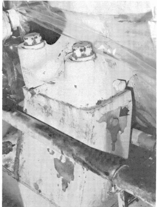
Figure 14. A View of a Pedestal Supporting the Low Pressure Stage of the Compressor Train. This Pedestal was Filled with a Special Mortar Comprised of Epoxy Liquid and Steel Shot in an Attempt to Increase Mass and Rigidity of the Support.
