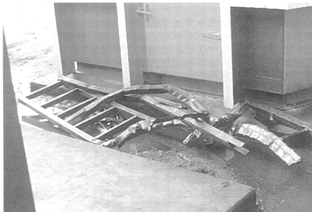
Figure 49. Mangled Remains of an Inspection Ladder That Was Left Within a Silo Combustor During Startup.
