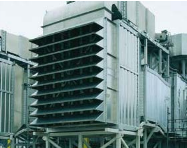
Figure 4. Weather Hood on inlet Filtration System (Offshore, 2009).
