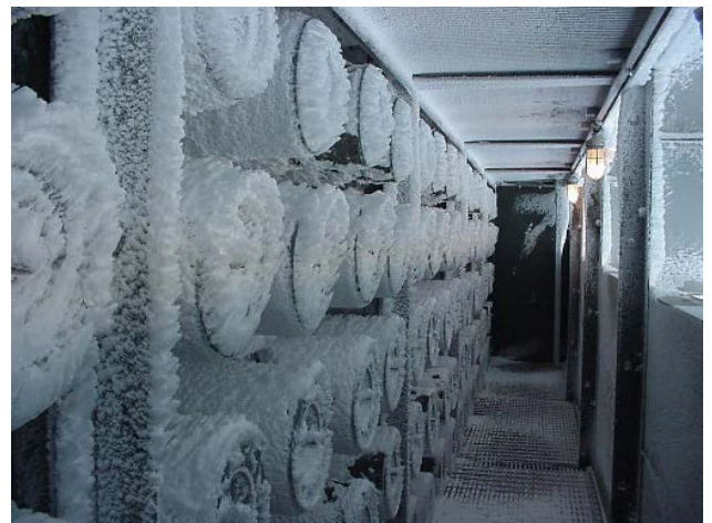
Figure 5. Cartridge Filters with Frost Build Up Due to Cooling Tower Drift (Wilcox et al., 2010).
