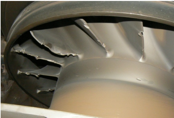
Figure 6. Fifth Impeller blade leading edge damage – June 2007
