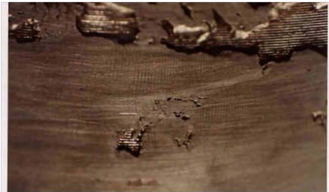
Figure 20 Close up of fatigue damage
