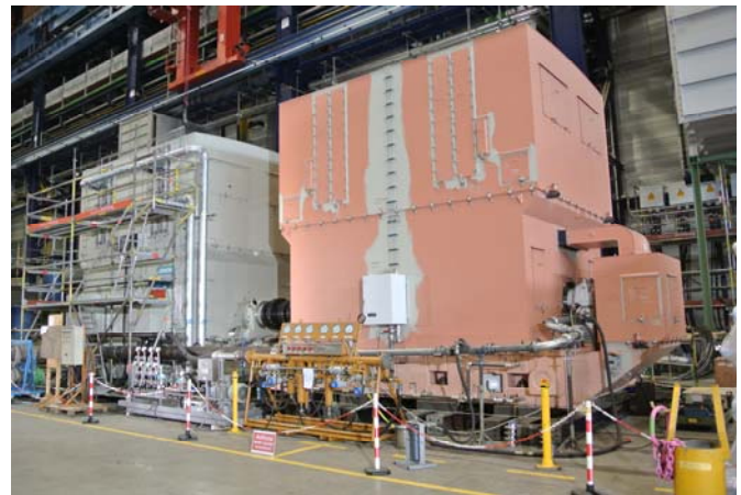
Figure 21. 78.7 MW Motor Generator Back-to-Back arrangement
