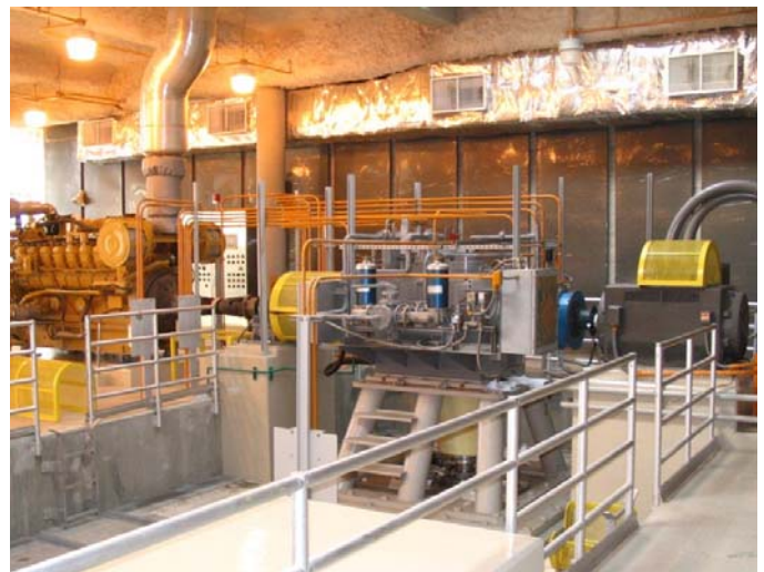
Figure 14. Water Pump System.
