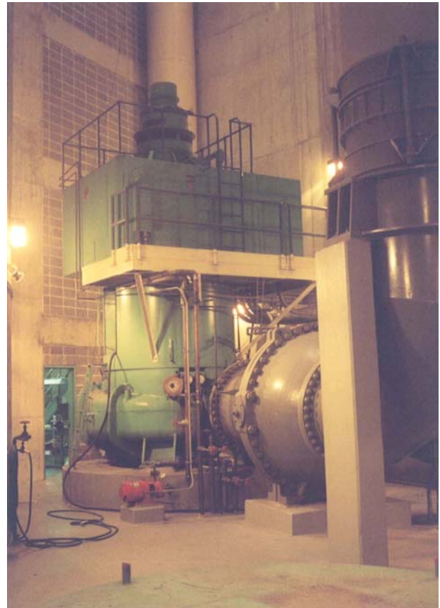
Figure 15. Vertical Motor - Pump System.
