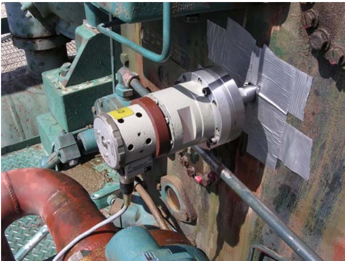
Figure A.10. Torsiograph on Oil Pump End of Compressor.
