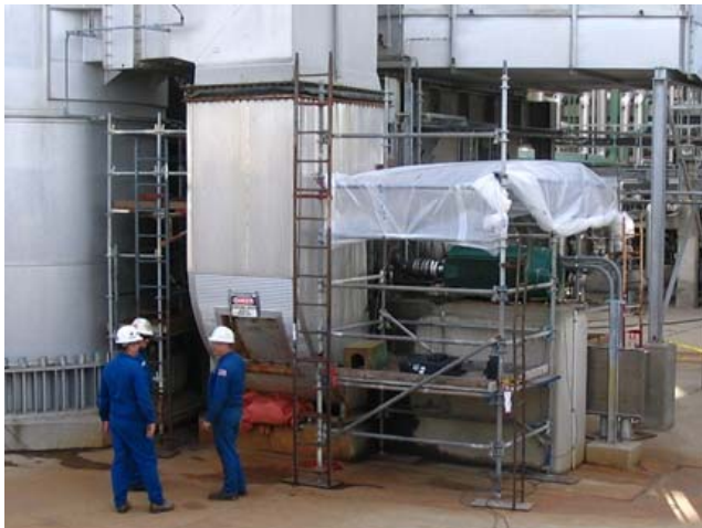
Figure 18. ID Fan and Motor.
