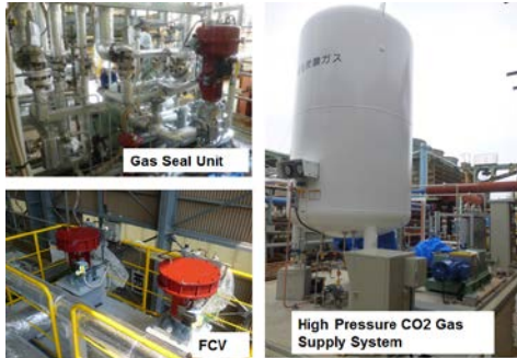
Figure 26. Upgraded Facilities for Super High Pressure Test
