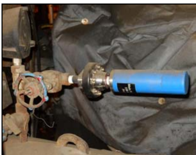
Figure 3. Tee Connection with Local Pressure Gauge (Vertical- Left) and Wireless Pressure Sensor with Battery Powered Transmitter (Horizontal-Blue).
