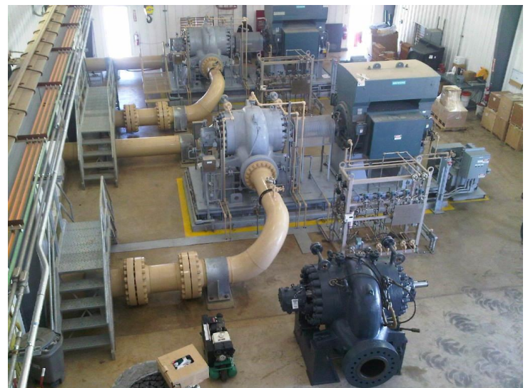
Figure 22. Pump Station (Courtesy Kinder Morgan)
