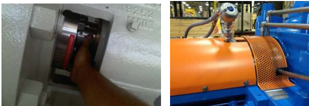
Figure 1: Unguarded shaft area vs. guarded
