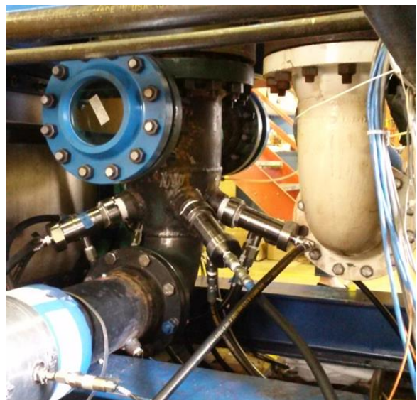
Figure 5. Installed Suction Piping with Sight Windows and Air Atomization Nozzles
