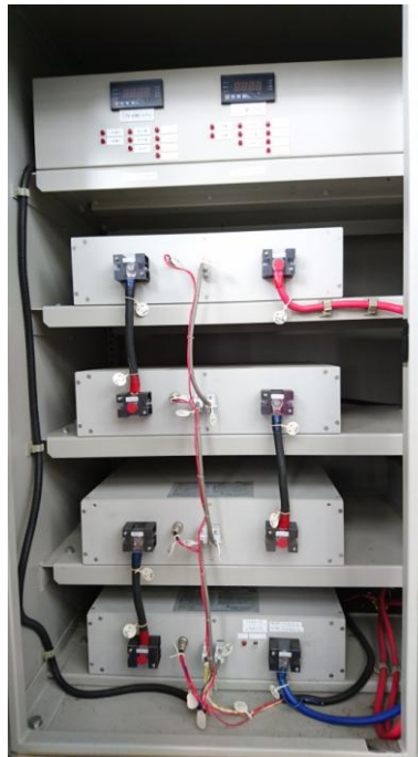
Figure 2. 14: Lithium – ion Battery 15 kW – 7.5 kWh in the CNES under study.
