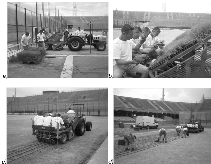
Figure 1: Work yard for the transplanting of single potted plants of bermudagrass in untilled soil.
