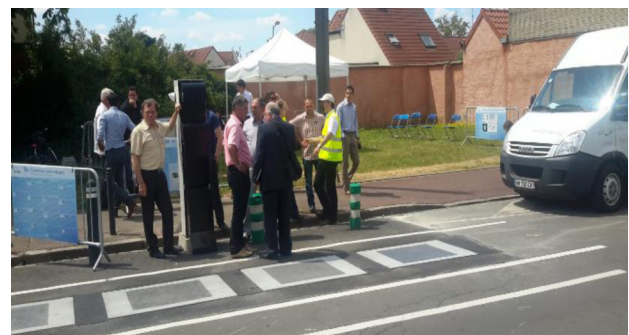
Figure 12. Dynamic inductive charging installed in Douai, France. (Source: FastInCharge project)
