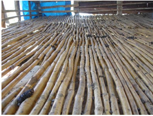
Dangerous bamboo flooring
