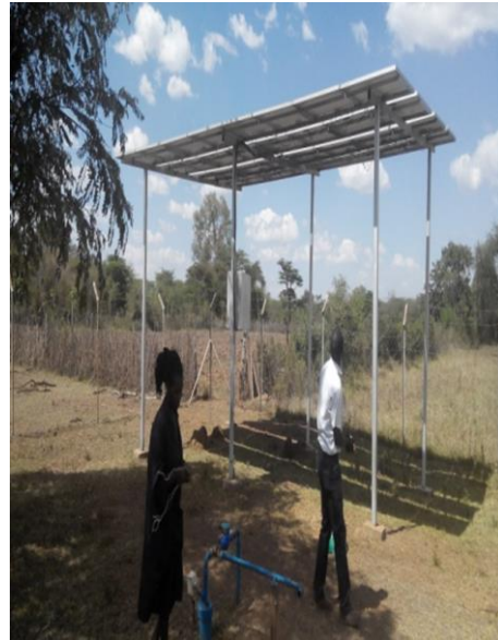
Photo 8: Chepchomus borehole supply water to 14 individuals' connections & one water kiosk
