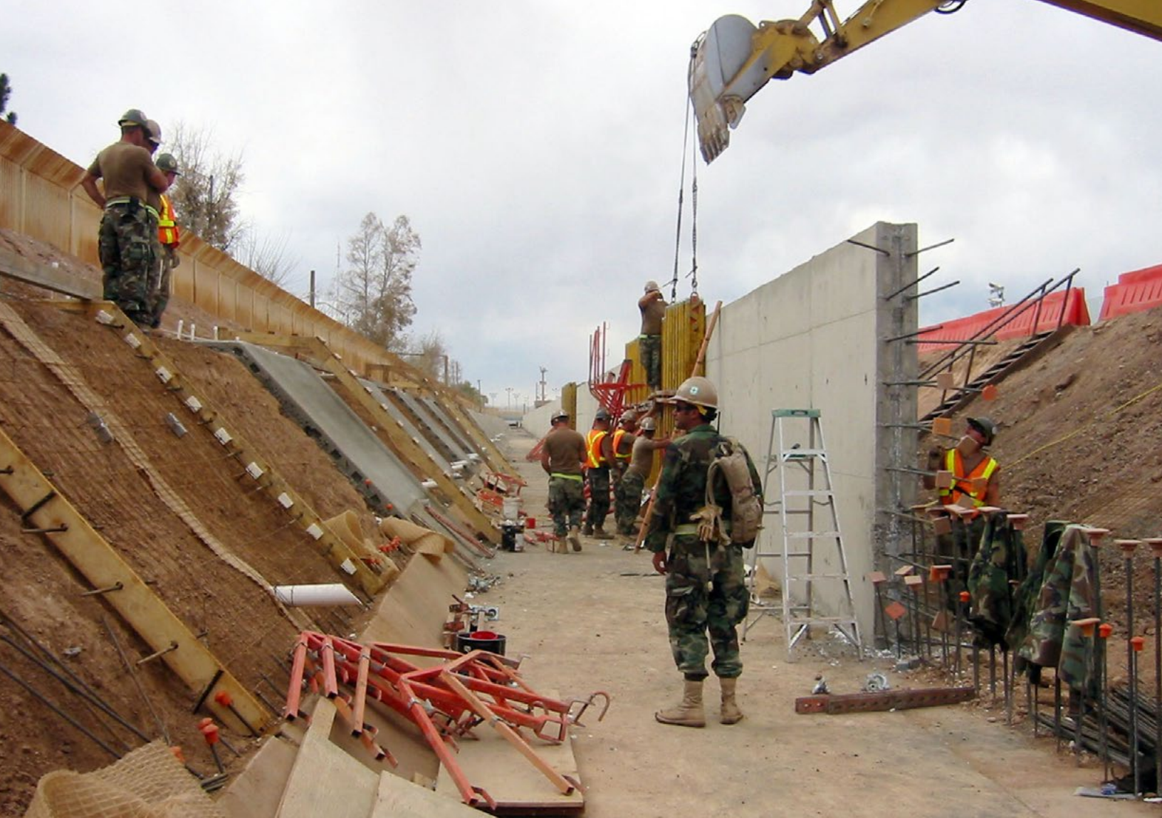
March 14, 2009, Naval Mobile Construction Battalions construct a concrete-lined drainage ditch and a 10 foot-high wall along the U.S. and Mexico border in Douglas, Ariz.
