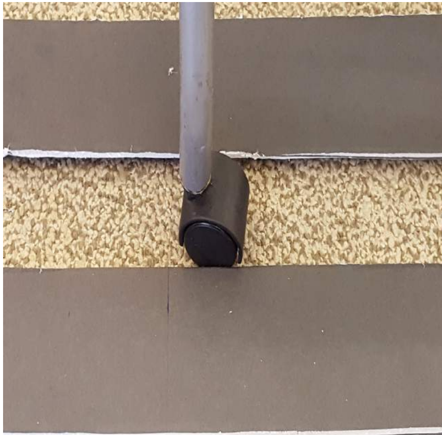
Figure 5. Caster wheels guided by a track low enough to leave with the help of an impact
