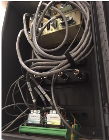
Figure 44. Inside of dyno control Box
