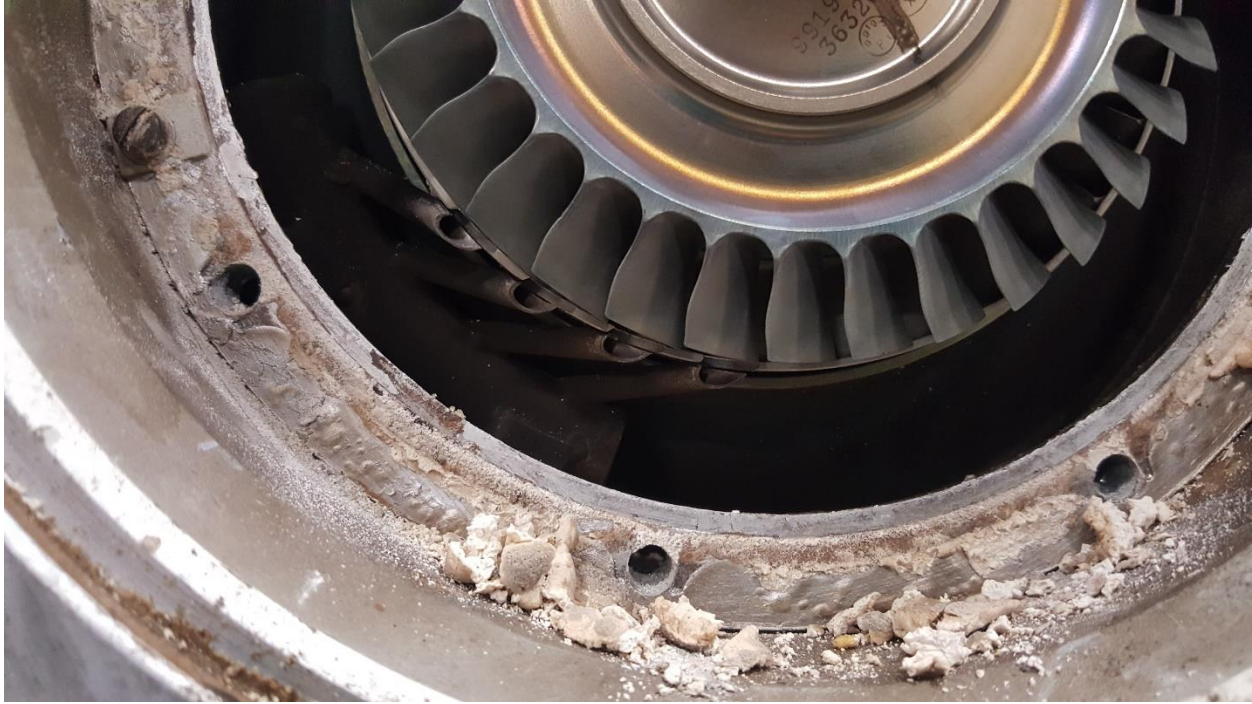
Figure 25. Air-start rakes at Stage 3
