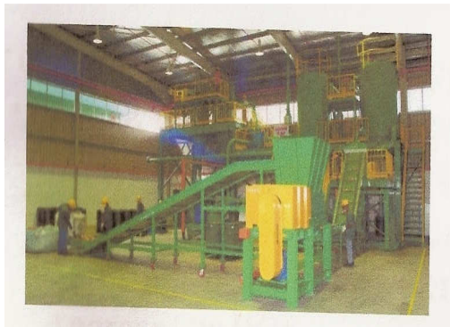
Plate 2.12: A crusher plant. (Source: Reclaimtek (M) Sdn. Bhd.)
