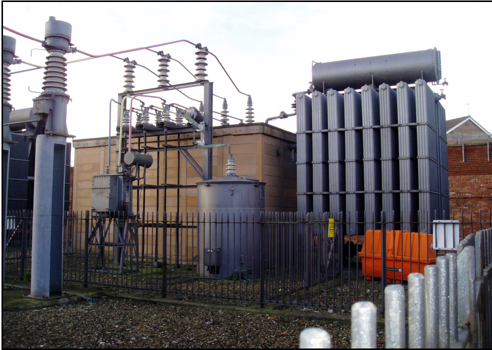
Figure 5.3 – Old transformer at Amberton Road
