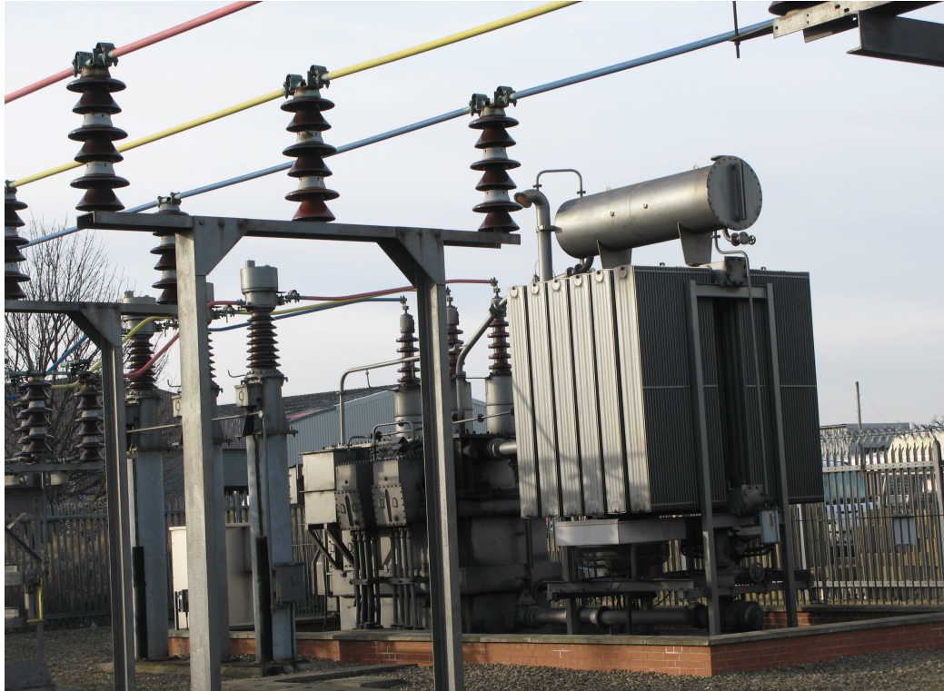
Figure 9.3 – Transformer and 66 kV busbar at Brenda Trading
