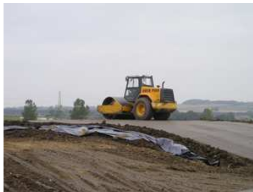
Figure 3.4 - Construction of a well compacted panel using a self propelled vibrating smooth drum roller, (Hughes, 2005).
