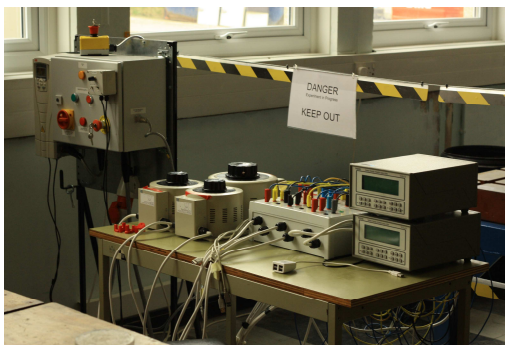
(e) Control and measuring equipments
