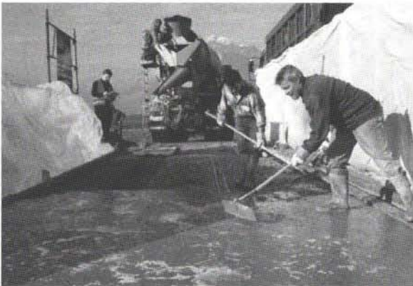
Figure 12: Overall view of the UHPFRC pouring on the bridge deck slab (Photo A. Herzog).
