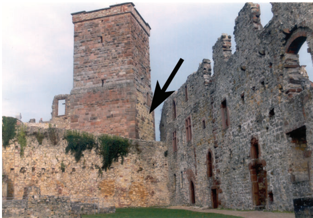
Figure 9. Picture of Rötteln Castle close to Lörrach (Schomann, unpublished data). See noticeable repairs on its eastern side (see arrow). Documents providing reasons for the repair do not exist.
