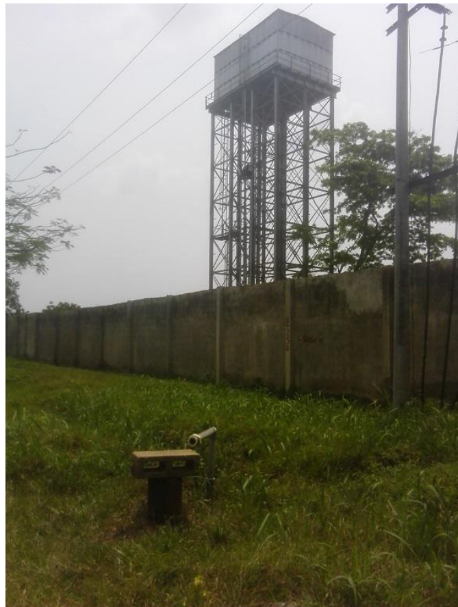
Fig. 2 A dysfunctional borehole close to an elevated water tank
