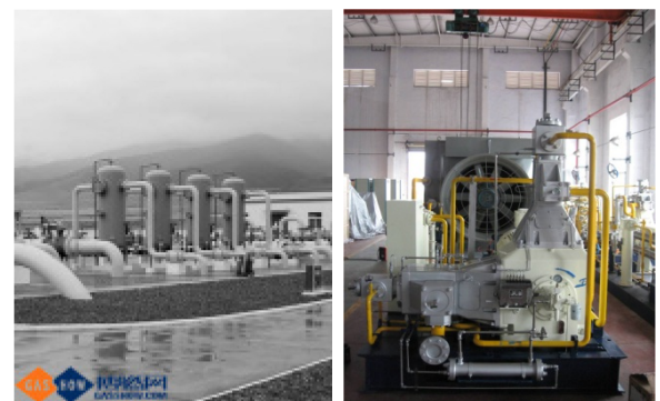
Figure 4: Hudong natural gas compressing station and compressor [7]
