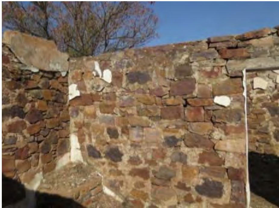
Figure 4.12: Interior of Motse 11.25 with the white plaster and the remnants of a fire place. (Photo: Author's own).
