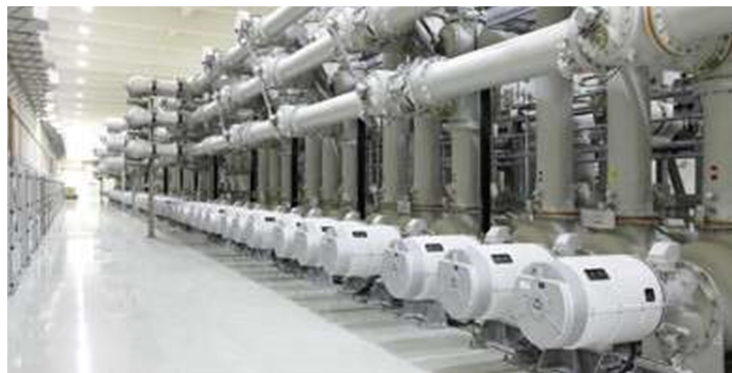
Figure 2.6: Gas insulated switchgear used in the industry [14].
