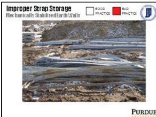
(c) Bad practice for reinforcement straps
