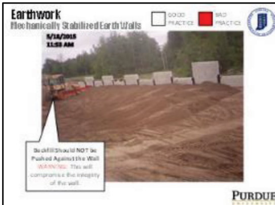
(e) Poor practice for MSE earthwork
