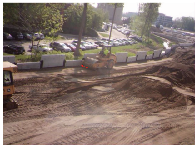
(c) Vibratory roller is too close to the wall
