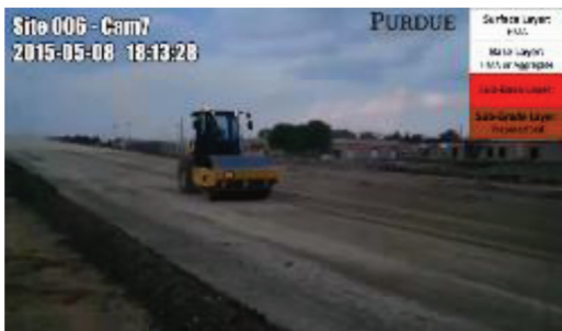
(e) 5/8/15 6:13 PM – Soil is compacted
