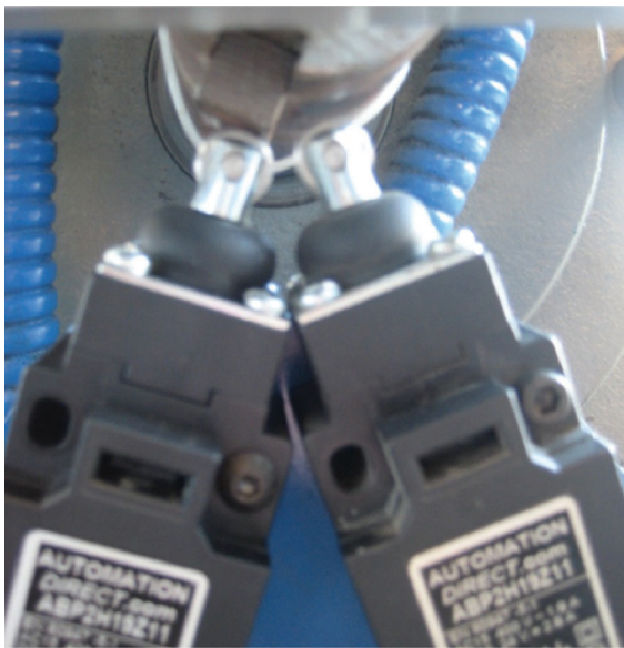
Figure 3.5 Original position limit switch engaged.
