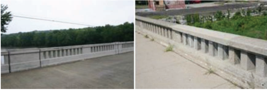
Figure 3.6 Concrete 6 railing (Rank 6).
