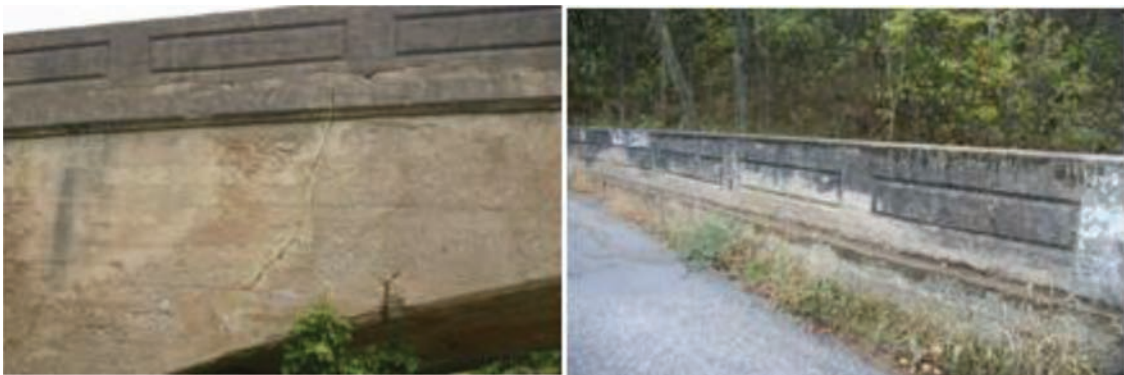
Figure 3.5 Concrete 2 railing (Rank 5).
