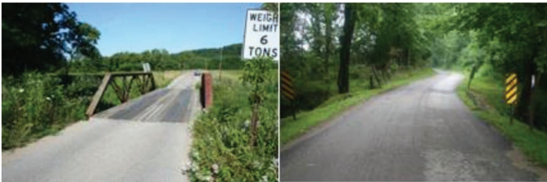
Figure 3.8 Bridges with no railing (Rank 8).
