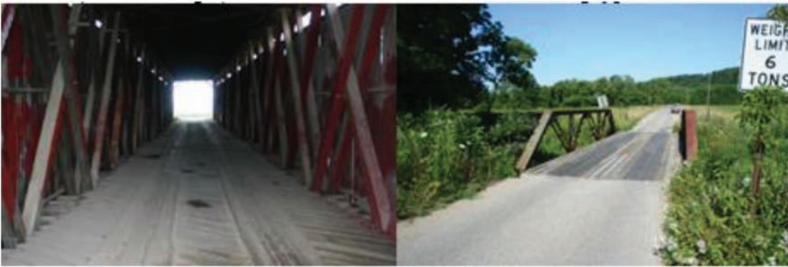
No Railing (35 bridges)
