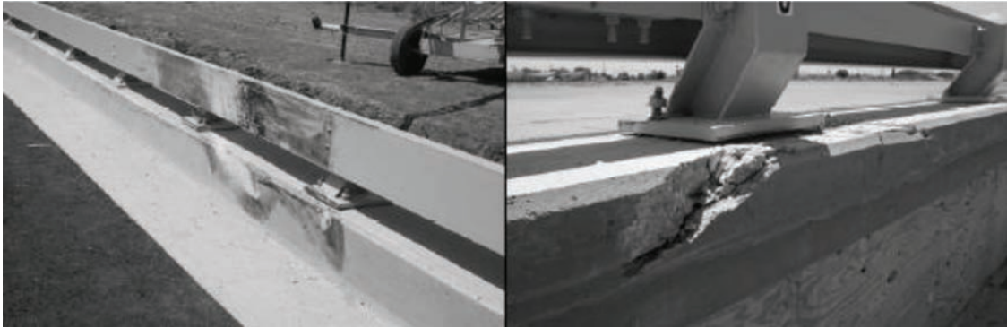
Figure 2.9 Test setup of the U.S. 281 railing after crash testing (Buth et al., 2004).
