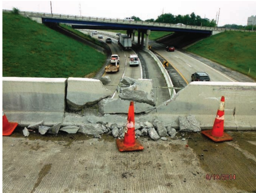
Figure 6.11 Nonsymmetrical impact failure (INDOT, n.d.).
