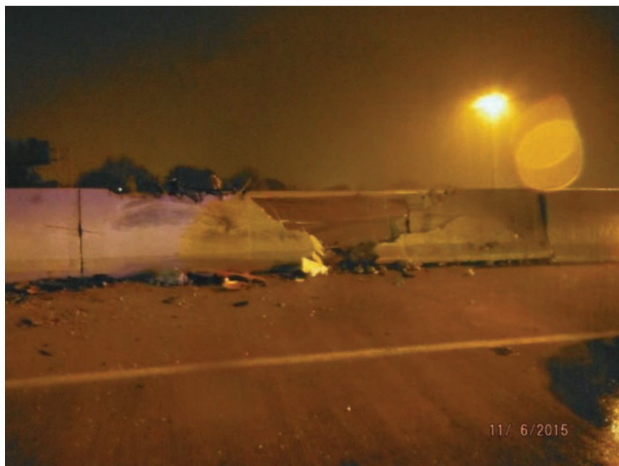
Figure 6.9 V-notch barrier failure (INDOT, n.d.).
