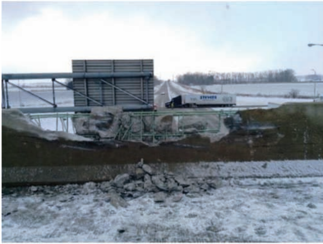
(a) Field Failure
