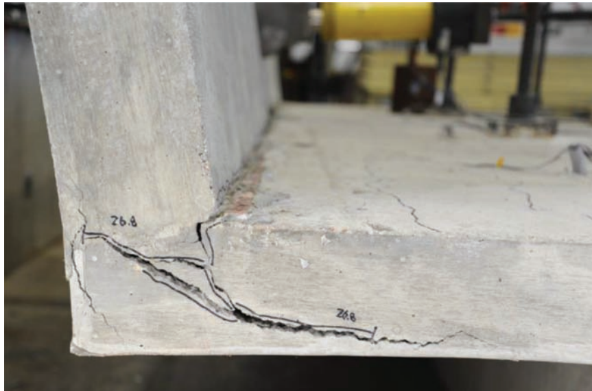
Figure 6.3 Joint shear failure (Specimen 1).
