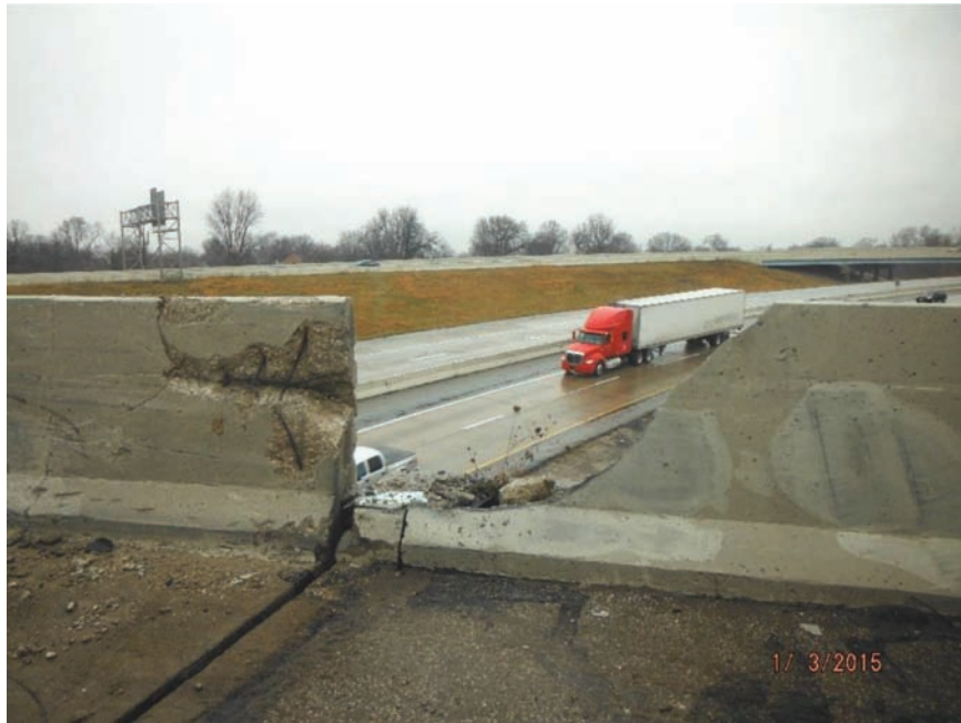
Figure 6.12 Nonsymmetrical impact failure (INDOT, n.d.).
