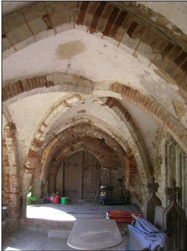
Fig. 3.7: View looking south through the corridor. Note the plastered brickwork of the corridor painted to imitate blocks of ashlar, best seen on the longitudinal ridge rib at the top of the image.
