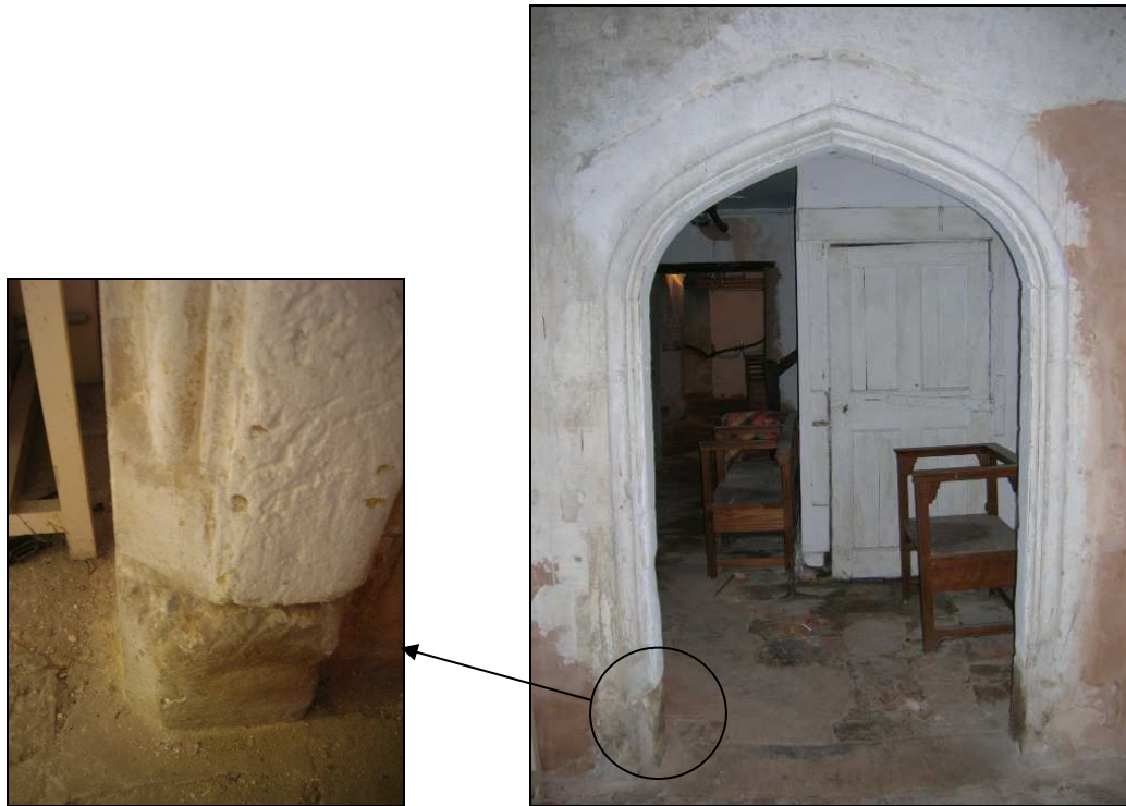
Fig. 3.57: The doorway in the southern chamber of the cellars, looking southwards. Note the roll mould decoration running around the doorway. At the bases of the jambs (the left image shows the eastern jamb) there appears to be a simple chamfer termination to the roll moulding and on the stone beneath a tapering to a second plain chamfer.
