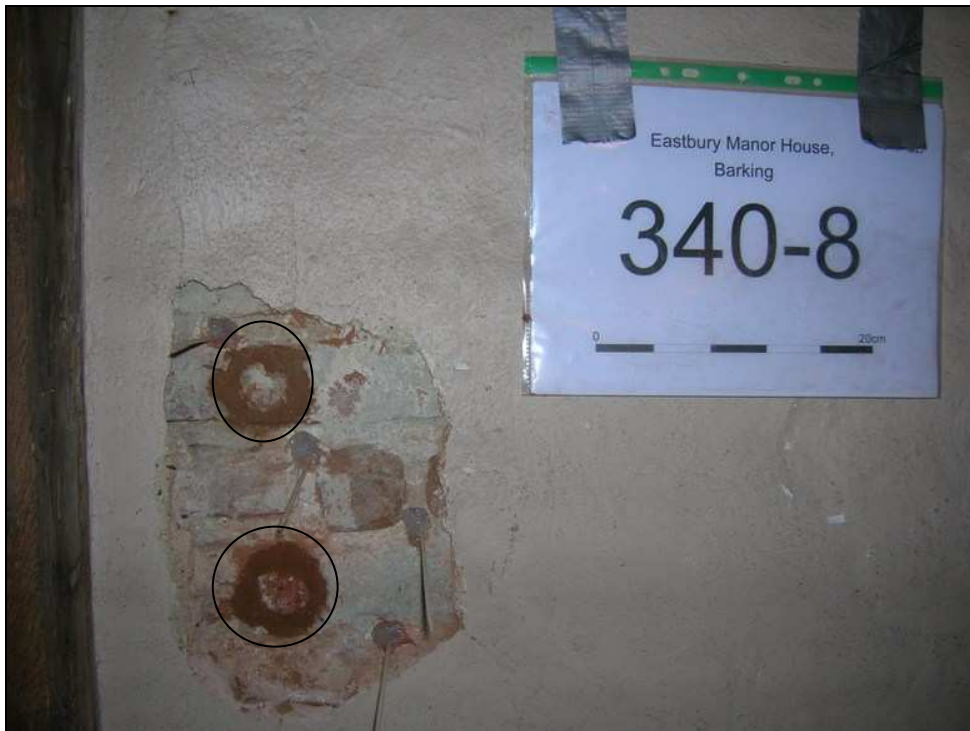
Fig. 3.22: The south western corner of the attic space where two samples were collected. The sample points have been circled. The scale bar is 20 cm in length. The image shows the wet mortar repair work shortly after sampling had taken place.
