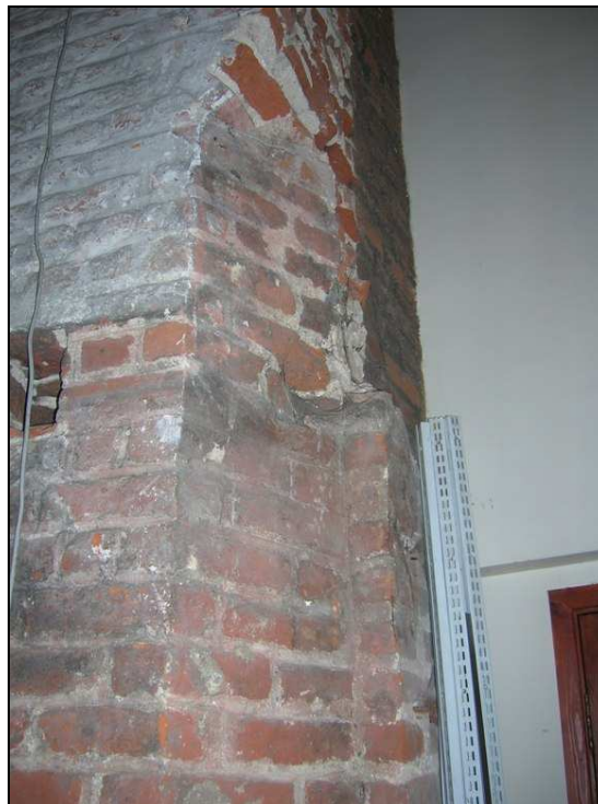
Fig. 3.32: Springing of a four centred opening in the wall of the building to the east of the Moot Hall. The height between the top of the opening and the holes in the wall suggest this was originally a window.
