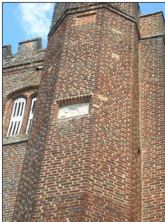
Fig. 3.115: The southern face of the stair turret. Note the weathered stone panel set at the second stage level and the blocked recess at the top of the turret, just beneath the string course.
