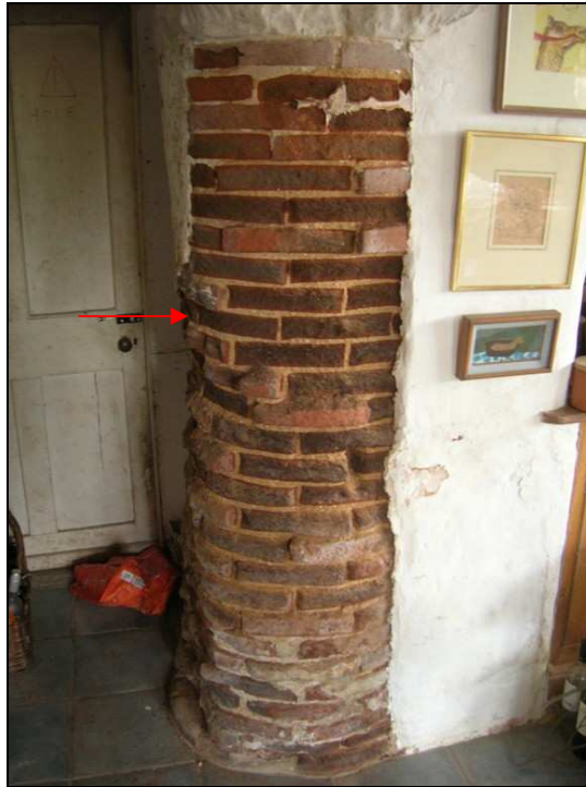
Fig. 3.14: The mid-12 th century medieval brick column that is thought to have originally been part of the infirmary. The arrow indicates the sampling point. Note that the pillar was originally of greater diameter but the outer surfaces of the bricks have eroded.
