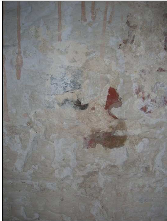
Fig. 3.58: An image focused on a small portion of the western wall within the cellar. Note the exposed fragment of orange colour brick located centre-right side of the image and the contrasting exposed fragment of a darkened, partially vitrified brick located centre-left.
