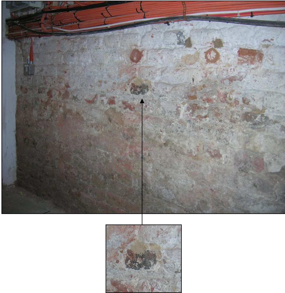
Fig. 3.16: The southern wall of the northern cellar. Occasionally, darker, vitrified bricks can be seen among the more standard red bricks. The bottom image shows a closer view of one such darkened brick.
