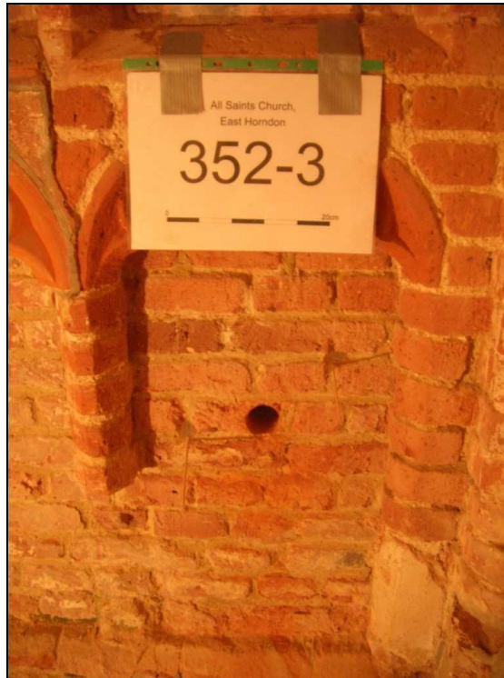
Fig. 3.88: The niche in the western wall of Thomas Tyrell's tomb niche. The label is covering the decorative cinquefoil corbelling located at the top of the niche. The irregularities of the bricks in this location contrast with the modern replacement material located in other areas of the niche, suggesting this is authentic 'Tudor' type brick. The scale bar is 20 cm in length.
