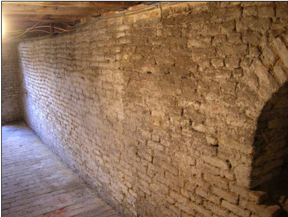
Fig. 3.62: The southern wall of the cellar, illustrating the extensive use of 'Flemish' type bricks.
