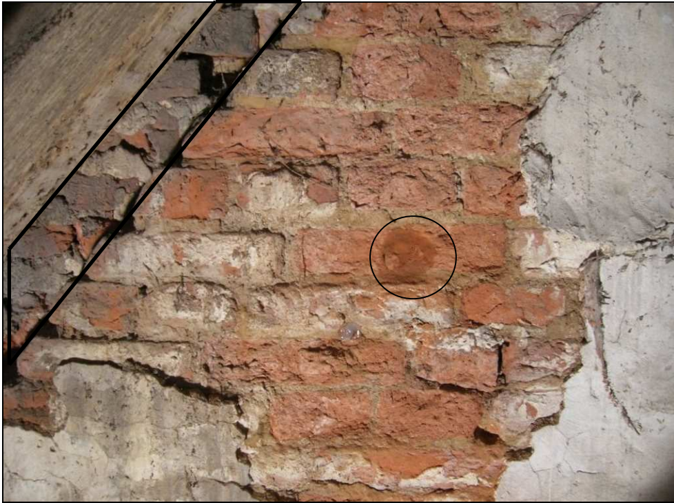
Fig. 3.123: The exposed portion of brickwork in the western wall of the belfry chamber. The rafter of the roof structure can be seen in the top left corner of the image. The sample point (circled) has been refilled and the mortar is still wet. Note that behind the outer surface of the wall, which terminates in a diagonal slope on the left side of the image, a second layer of brickwork can be seen (outlined in the image).
