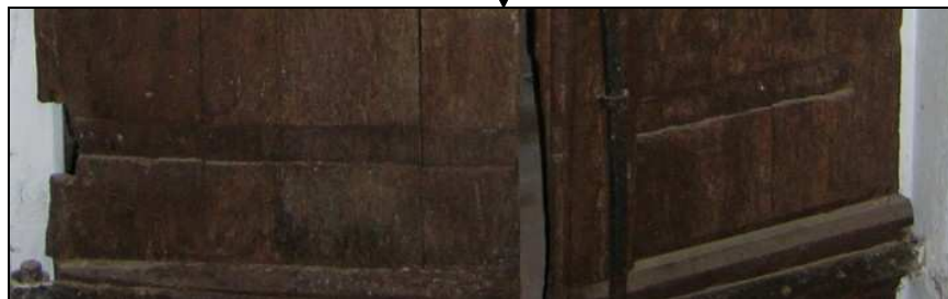
Fig. 3.56: The door and doorway between the north and south cellar chambers. The top image shows the north face of the door. Note that at the bottom of the present door there is a groove which runs across both leaves for an original hinge strap. There is also a niche on the left side of the image which was the location of the hinge loop to sit on the wall pintle.
