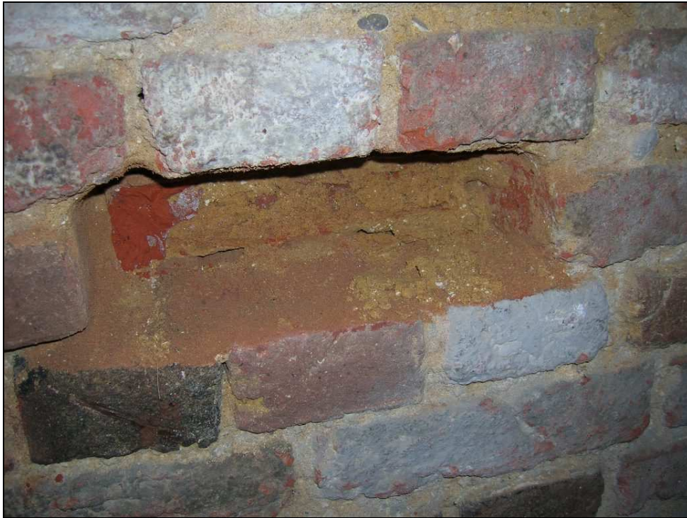
Fig. 3.106: The space where the sampled brick was located. The mortar surrounding the brick was drilled away before the entire brick was removed so that a sample could be taken from the rear surface to reduce the aesthetic impact.
