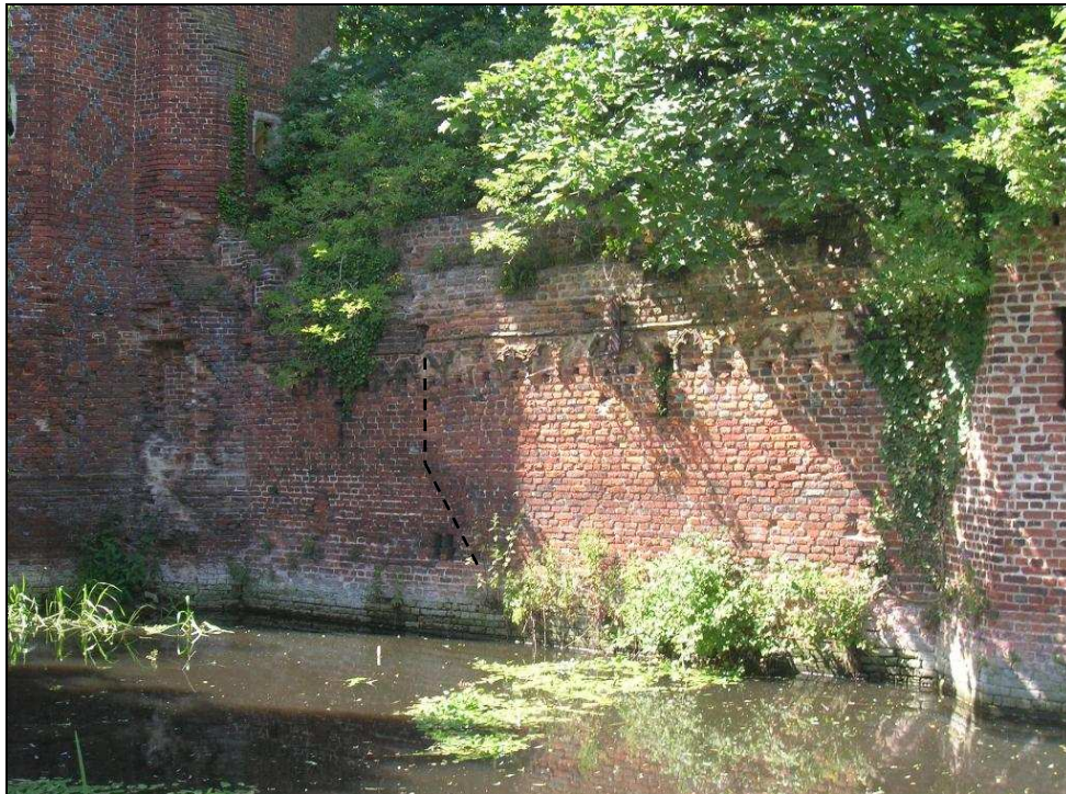
Fig. 3.46: The wall attached to the east side of the gatehouse. The dashed line represents the approximate location of the transition from high quality craftsmanship (to the left of the line) and poor quality craftsmanship (to the right of the line).
