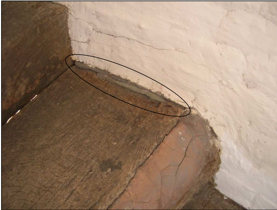
Fig. 3.17: Timber treads of the newel staircase inserted into the encasing brick wall. Note the use of grey slate (circled) to wedge the timber into place in the wall socket.
