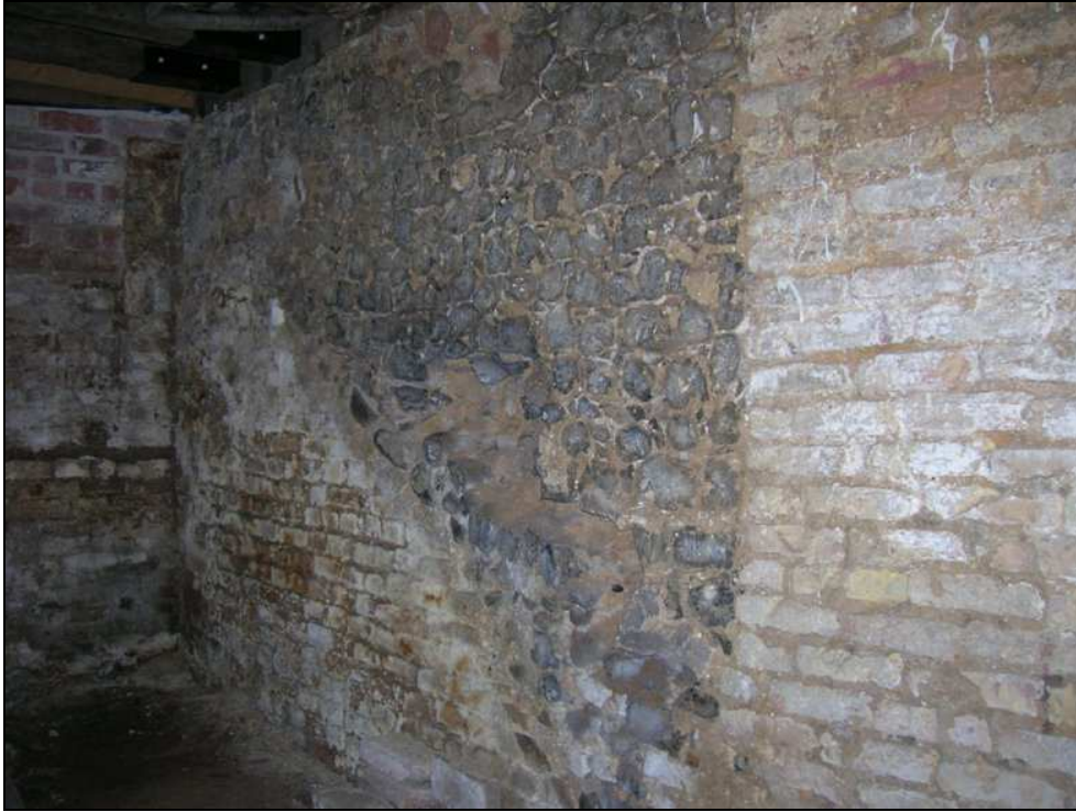
Fig. 3.63: The north west corner of the cellar showing the triangular segment of septaria in the wall. This feature is thought to be the remains of a ramp that served the shop above the cellar.
