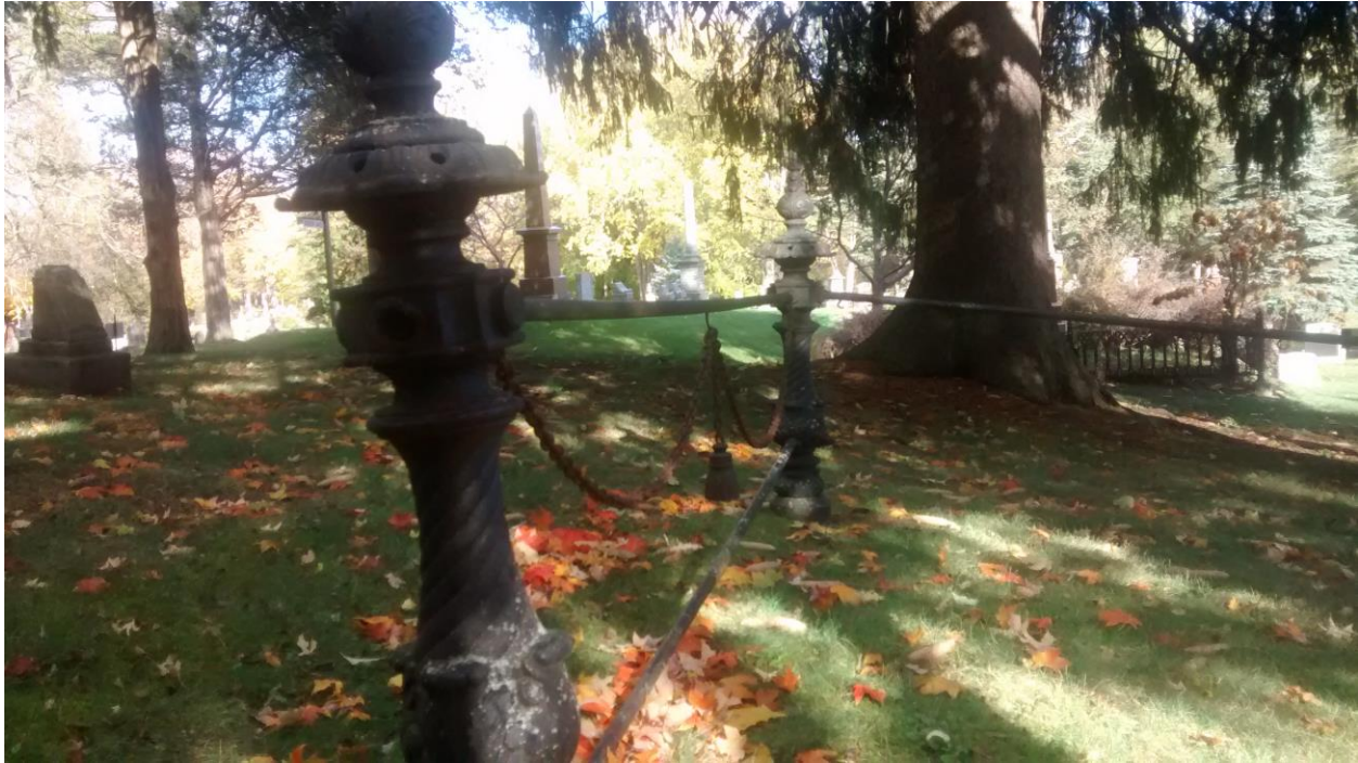
Plate 3 - A rusting iron fence. Though it is certainly worse off now than it would have been in the nineteenth century, with their tendency to rust and the difficulty mowing around them, one does understand why Nicol objected to the fences.
