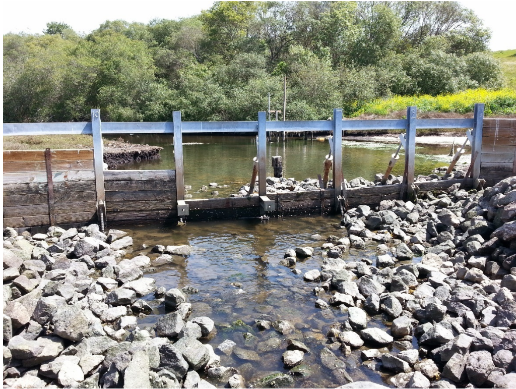
Fig. 2. South water control structure completed December 2009. Facing east looking into North Azevedo Pond from the main channel
