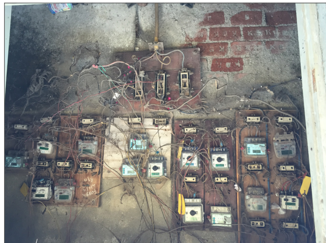
FIGURE 14: ELECTRICITY CONNECTIONS INCLUDING INDIVIDUAL AND “SHARED” CONNECTIONS IN A SLUM IN MUMBAI
