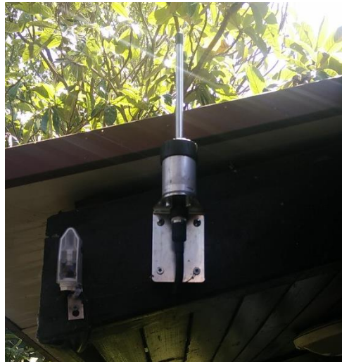
Figure 40 Antenna in N-building
