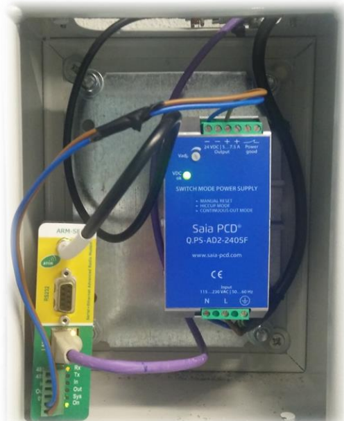
Figure 38 Installation N-building GECAD
