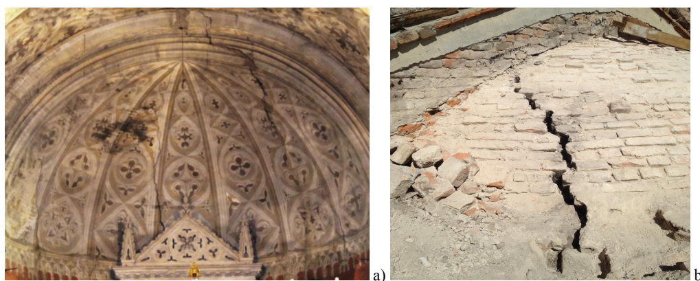
Figure 5: Crack pattern of St. Bassiano apse: a) internal and b) external view under the roof.
