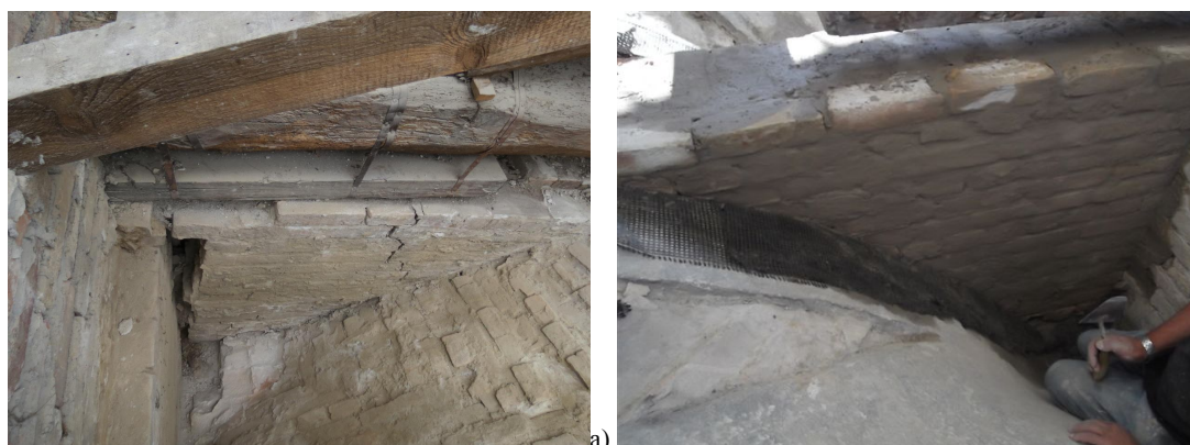
Figure 11: St. Bassiano church nave: a) damaged ribbed wall above a masonry vault and b) repaired ribbed wall and interlocked with the lateral walls
