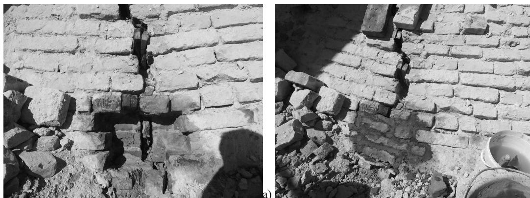
Figure 9: St. Bassiano church apse: cracks repair with “scuci-cuci” technique (literally, a technique of unstitching/stitching the damage masonry); before (a) and during (b) reparation
