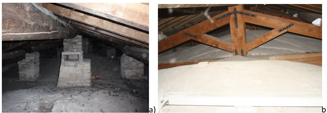
Figure 12: St. Bassiano church nave: a) old wood roof structure loading the masonry vaults and b) new wood roof structure with trusses
