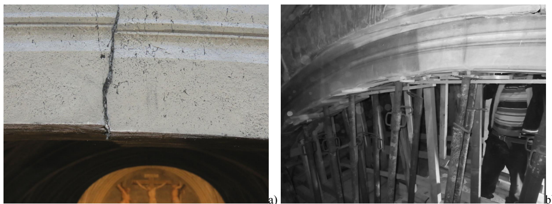
Figure 13: St. Bassiano church main arch between the nave and the apse: a) vertical sliding in the key before intervention and b) displacement in the original position with props
