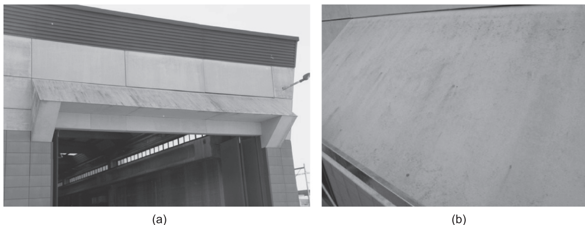
Fig. 11a–b. Heavy soiling deposits on the protection canopy (silica-calcium cladding).
