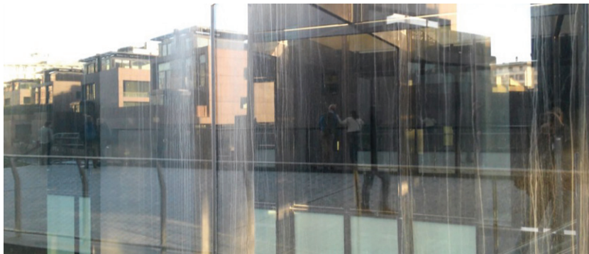
Fig. 1. Example of significant water stains on a facade, caused by lack of maintenance action.
