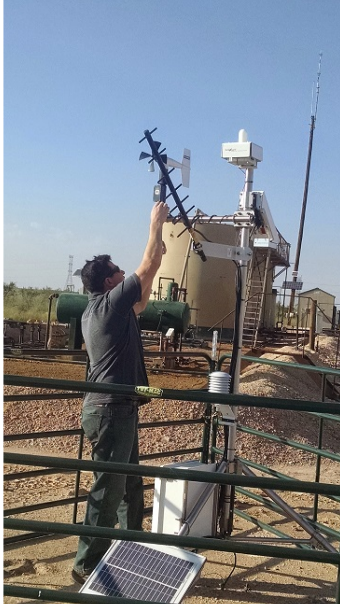
Fig. 5-8. Alignment of satellite communication antenna – Rooke 2014
