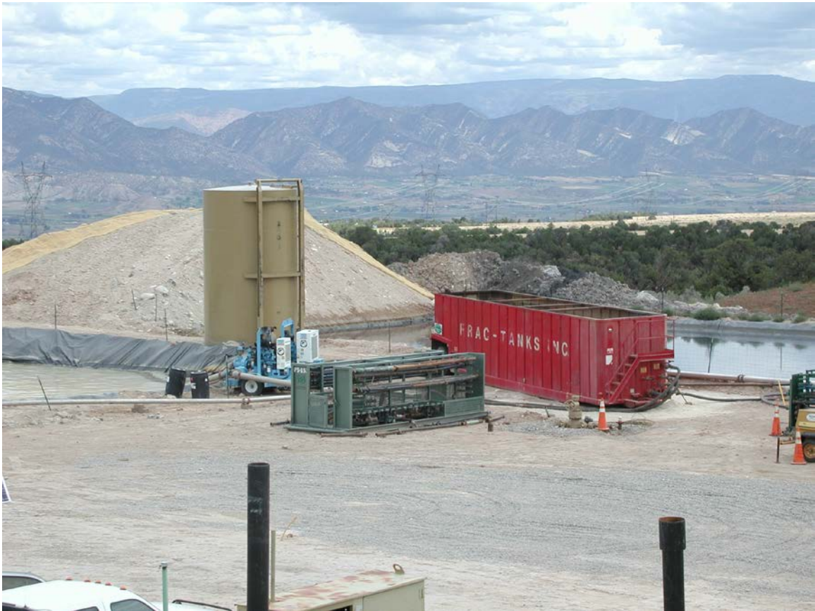
Fig. 2-1. Fracking pad with well head
