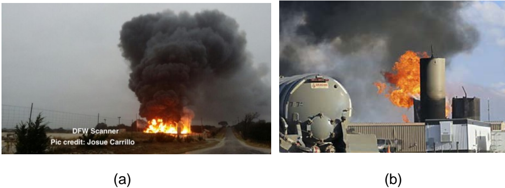
Fig. 1-14. Fracking batteries on fire (a) Texas, (b) North Dakota. Both fires were caused by lightning strikes.
