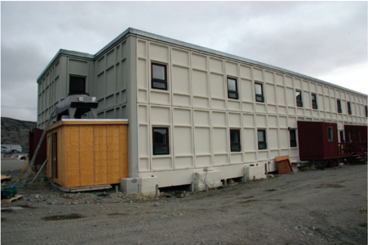
Figure 10.14 Building S385 in Kangerlussuaq suffered differential settlement of approximately 35 cm in its southeast corner after power was cut to an artificial cooling system installed below the building (photo by Thomas Ingeman-Nielsen).
