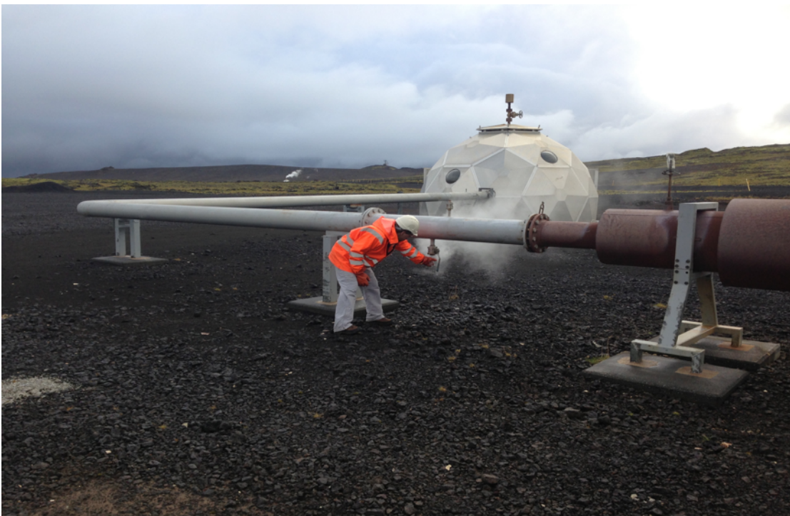
Figure 17: Geologist at geothermal wellhead, Hellisheiði, Hengill.
