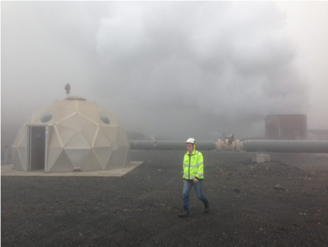
Figure 16: Geologist at geothermal wellhead, Hellisheiði, Hengill. The wellhead is the igloo like structure to the left of the picture. Following the thick pipe rightwards, there is an additional segment wedged between two pipe sections. The separator is attached here to access fluids. In the background to the right is the silencer.
