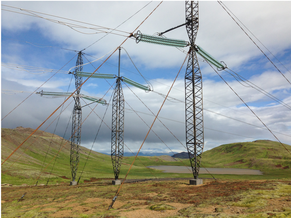
Figure 38: Pylons corroding at Hengill.
