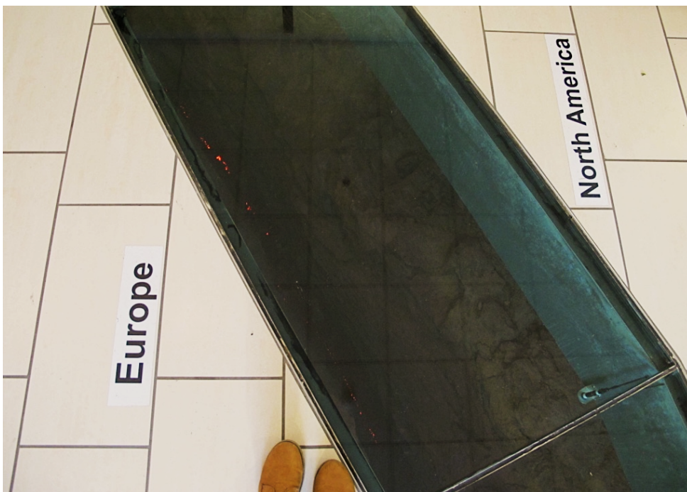
Figure 26: Fracture in Mall, Hveragerði.
