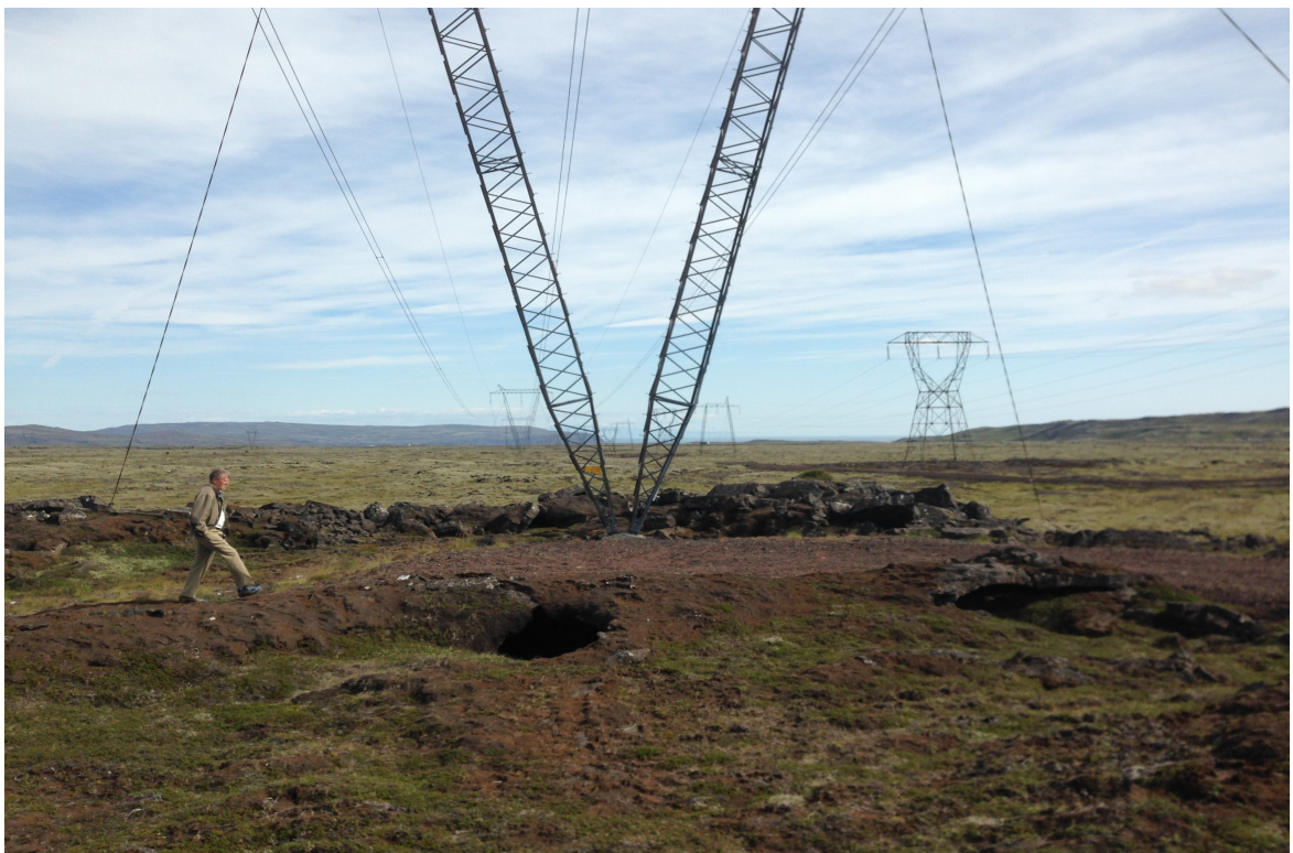
Figure 37: Björn noting Pylon corroding and lava damage at Hengill.
