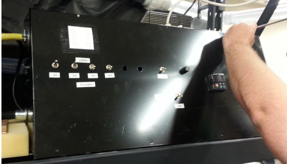
Figure 11. Original Manual Control Panel.
