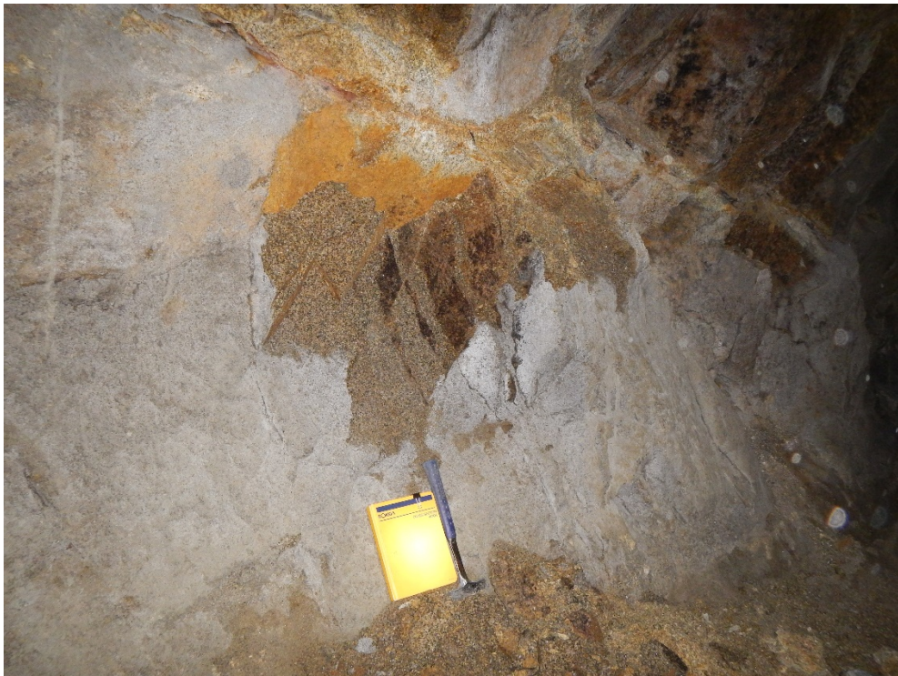
Figure 23: Weathering Grade IV observed at UMEC.
