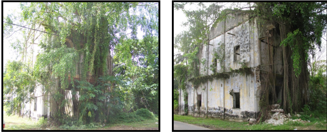
Fig. 1.4: Dilapidated buildings at Papan earning it a ‘ghost town’ status (source: author)
